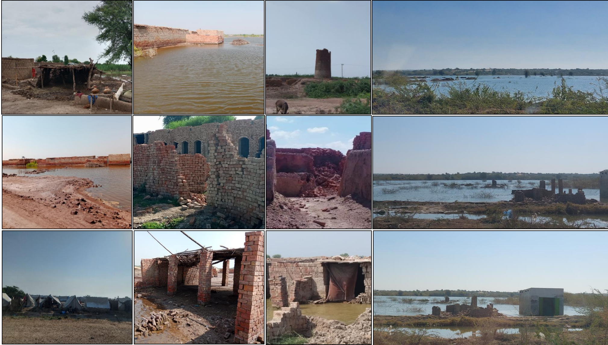
Damage to Brick Kilns and Worker Residences in MirpurKhas, Sanghar, Tando AllahYar and Umerkot Districts
